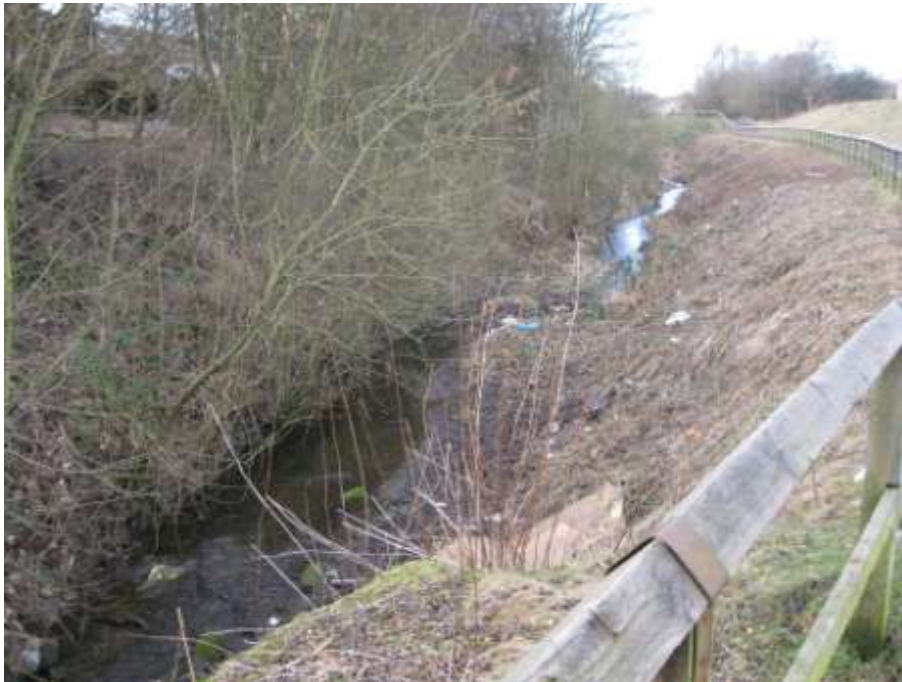
Final section of channel towards Pinxton Arm Junction and Codnor Park Reservoir, in deep cutting to provide flood route for Codnor Park Reservoir
