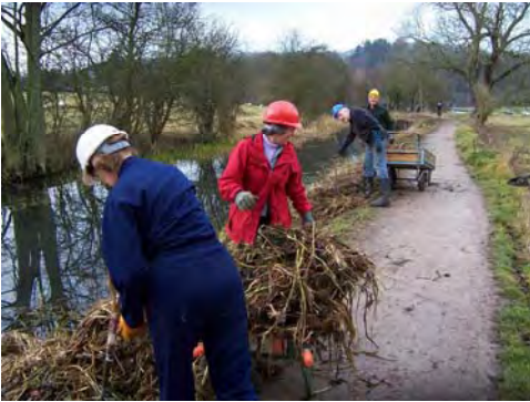
Volunteers work at weekends to clear vegetation from the canal channel, this work is vital; it must be repeated annually to allow the horse-drawn boat to navigate the canal
