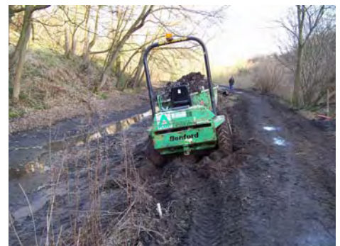
Lengths of the canal occasionally require draining to deal with major leaks.
