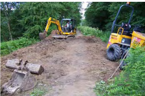
Tow path maintenance and dealing with small leaks are an ongoing maintenance liability
