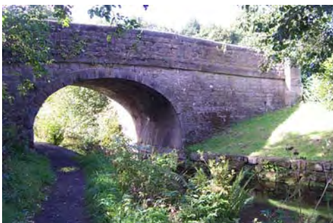
Hump-backed stone bridges took the few pre-existing roads and farm tracks across the Canal. All of the six original bridges on the Derwent Valley section survive.
