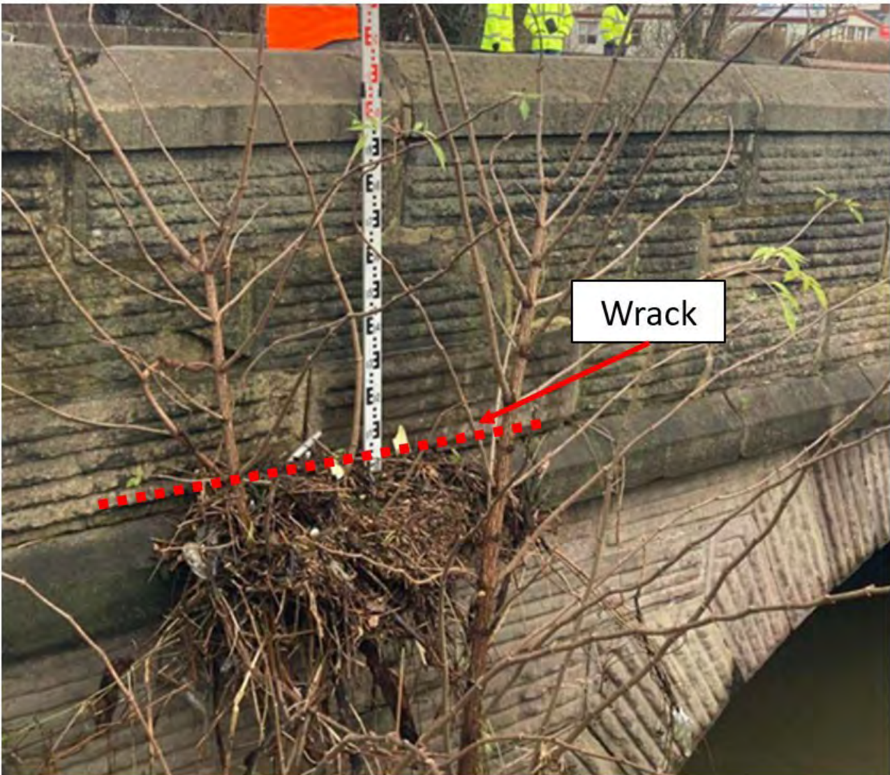
Figure 7-22: Wrack mark on the upstream face of Derby Road bridge. Source from the Environment Agency.
