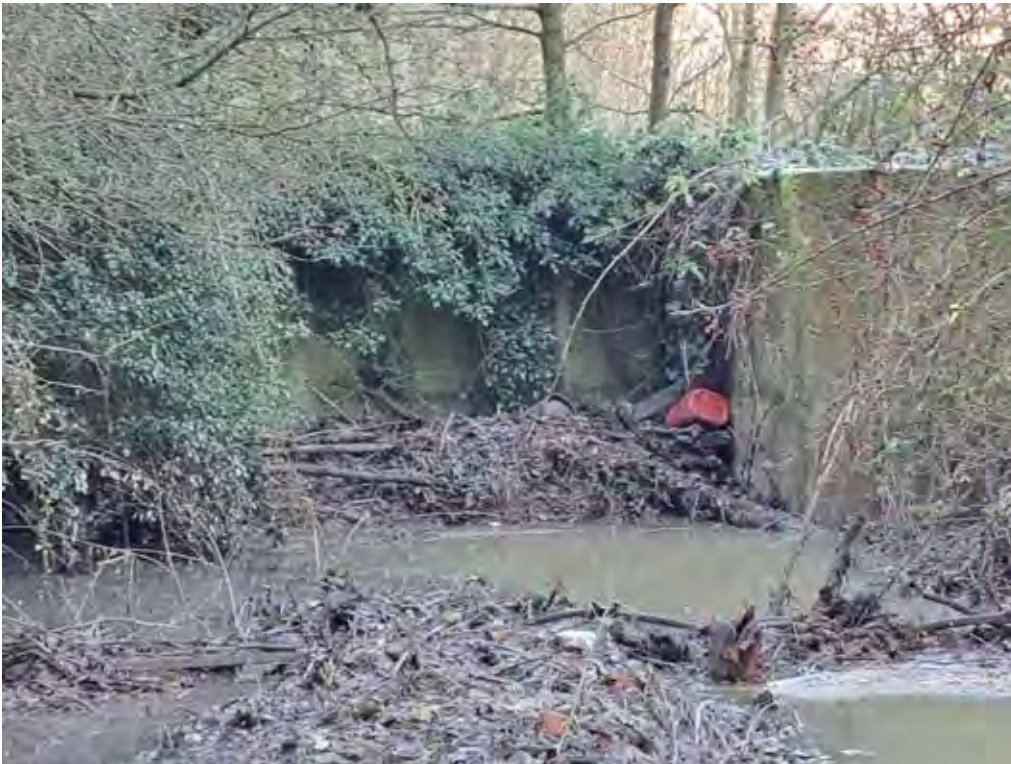
Figure 4-33: Debris blockage at Smithy Brook culvert inlet (upstream of Smithy Brook Road).
