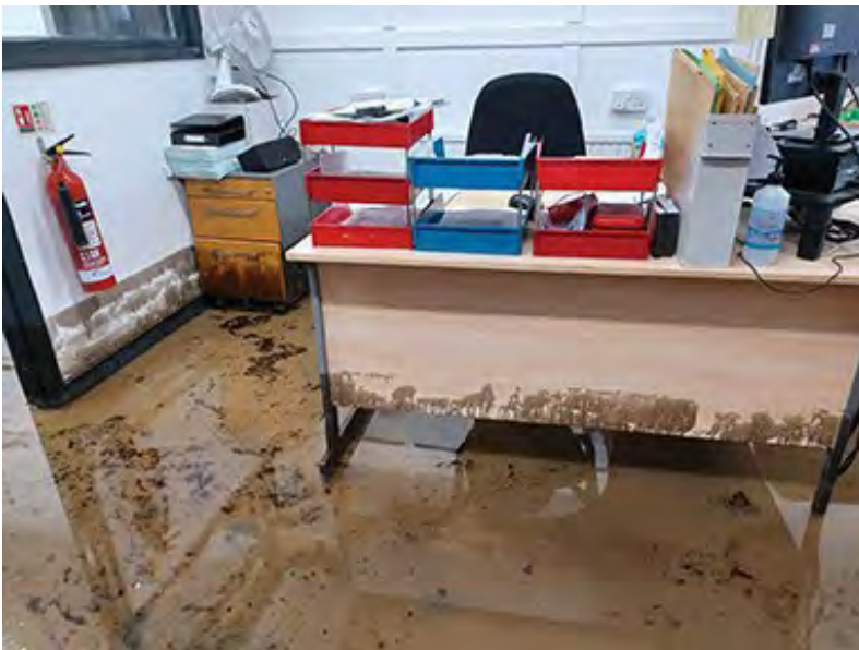
Figure 4-56: Interior of Eckington Depot affected by flooding because of Storm Babet.
