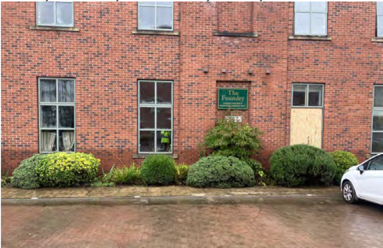
Figure 4-45: Photograph of watermarks reaching over 0.5m on The Foundry building, Camlough Walk taken in the aftermath of flooding.
