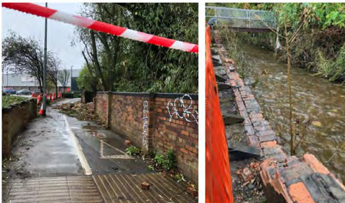
Figure 4-24: Collapsed walls as a result of the overtopping of Holme Brook (left) and the Hipper (right).
