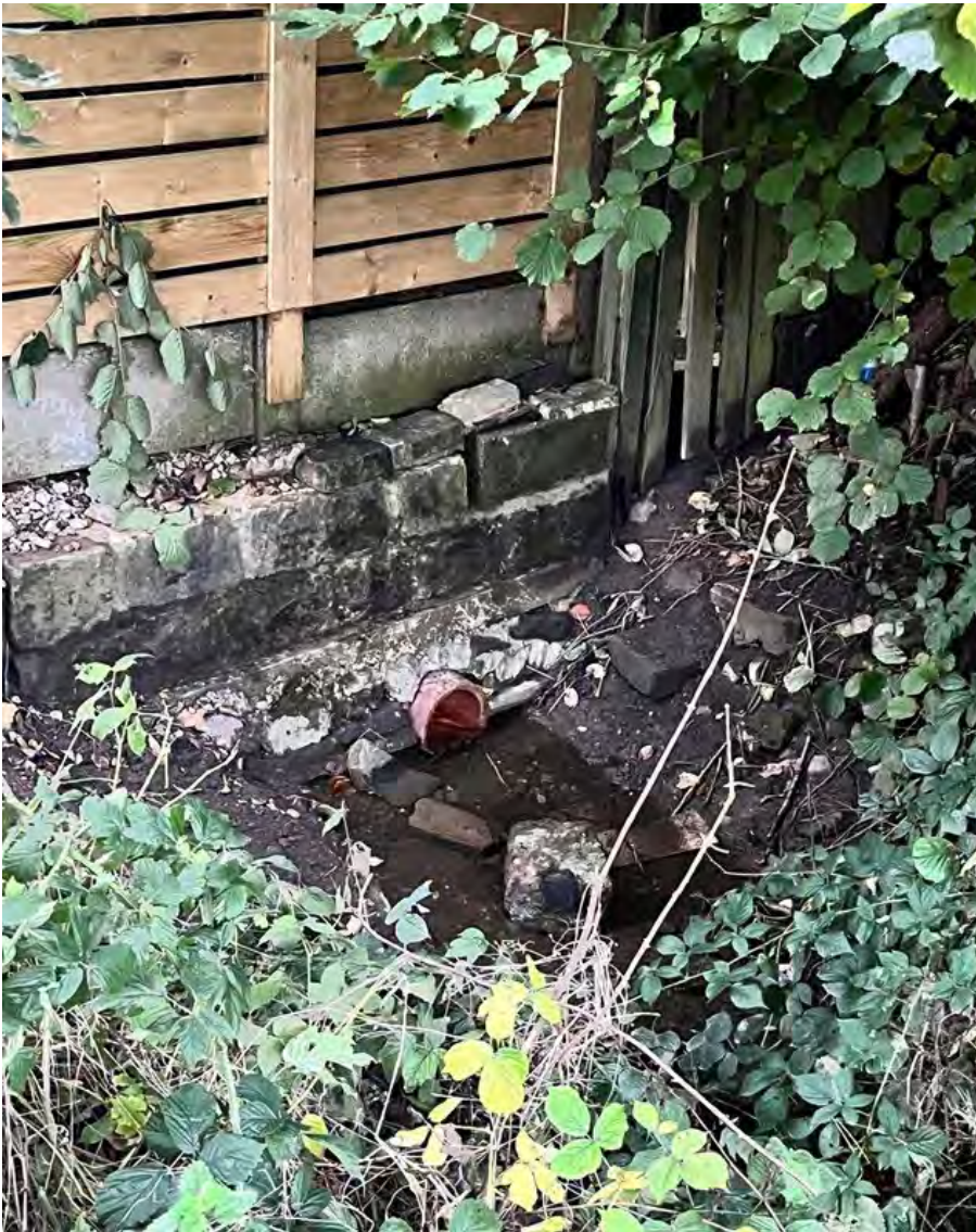
Figure 3-4: The culvert inlet of the watercourse which flows southwards parallel to Lilac Way.
