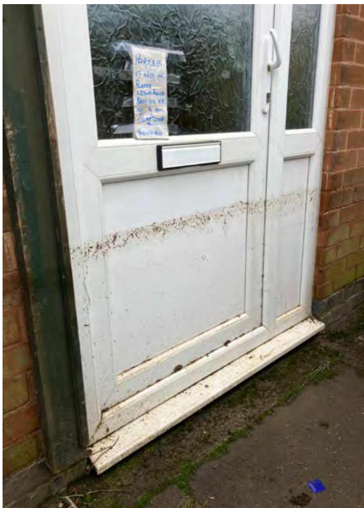
Figure 3-9: Flood water line on property door.
