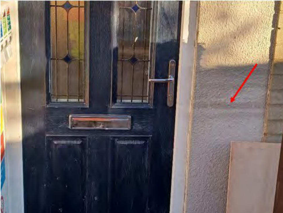
Figure 3-54: Flood water marks about halfway up the door and wall of a property in the community marked by a red arrow.
