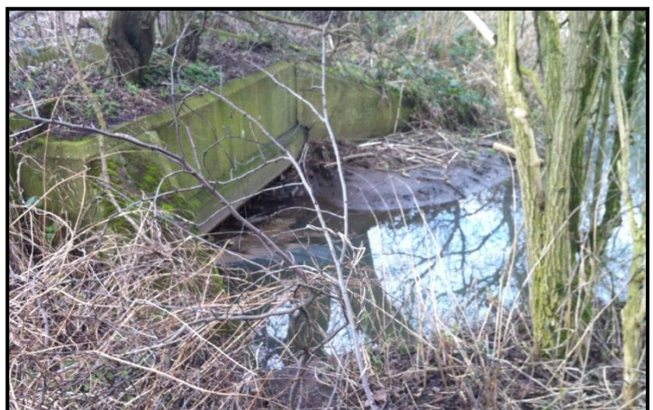
A silted box culvert
