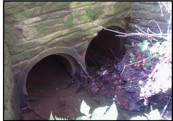
A partially obstructed culvert
