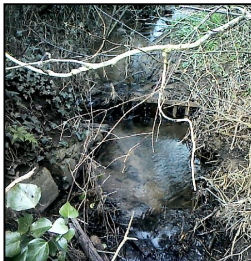
A partially obstructed trash screen
