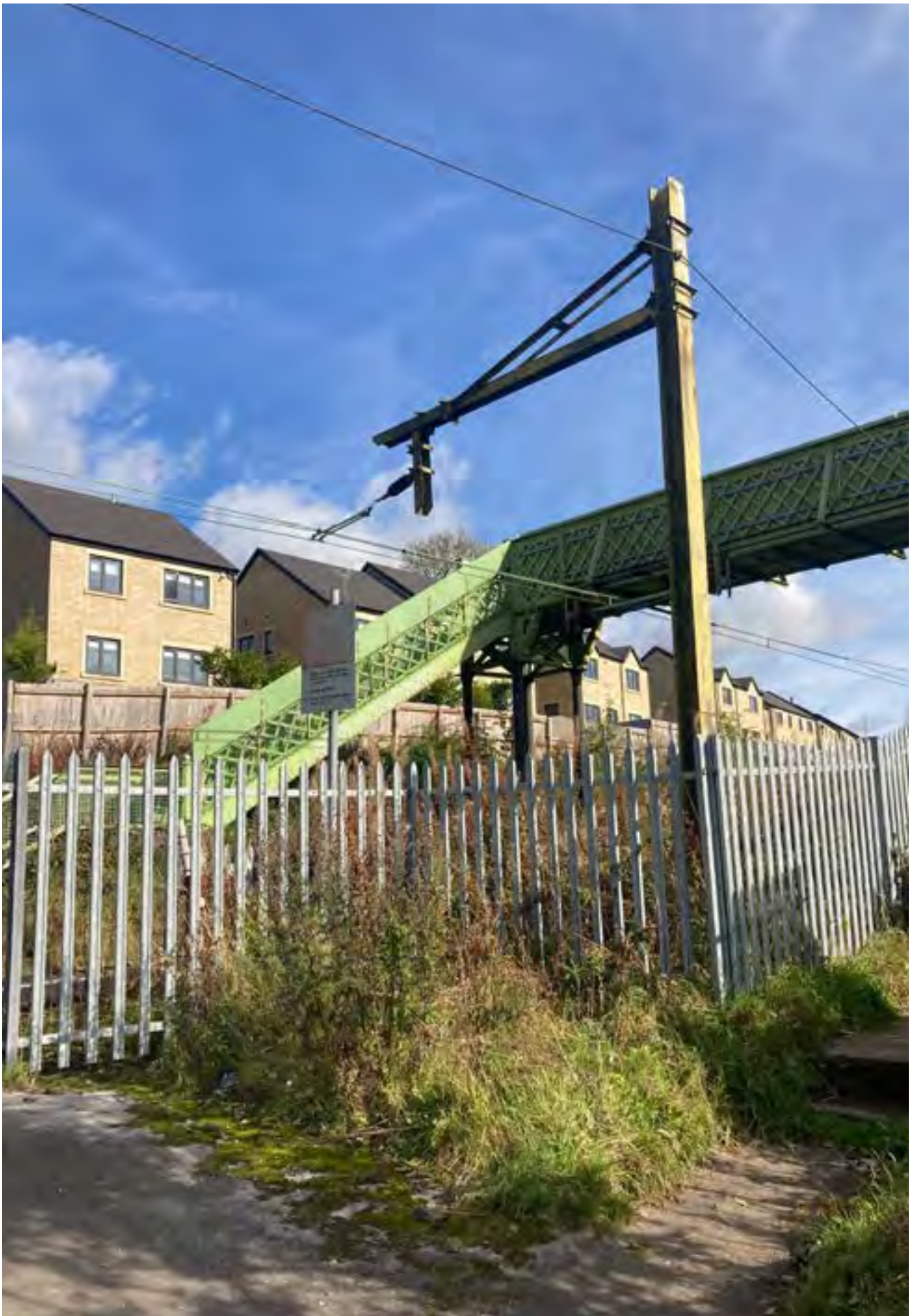
Figure 40: The existing footbridge which provides access over the railway line on Dinting Lane
