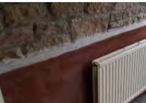
The walls were rendered on top of the membrane, using coloured renders
