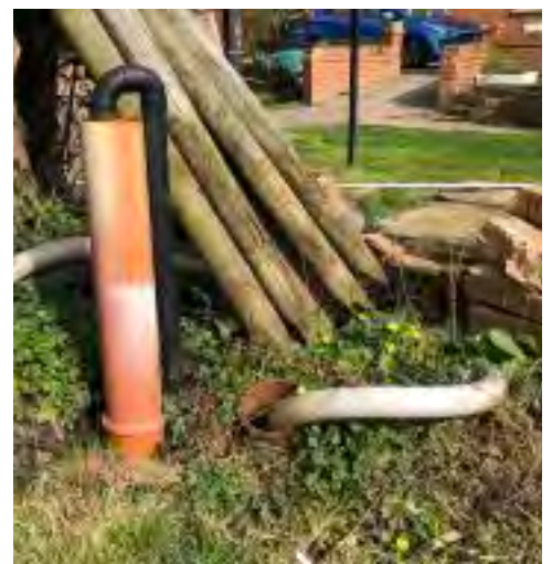
Rainwater runs through a series of French drains into a large sump into which a strong pump is fitted which pumps the water outside the garden boundaries.
