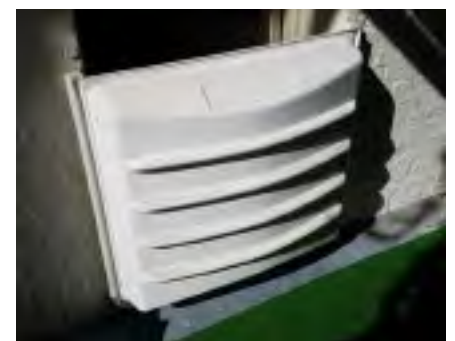
Flood barrier on the back door.
