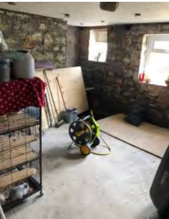
The basement room previously housed the kitchen and was extensively flooded to a depth of 5 feet.
