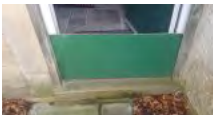
Home-made wooden ‘flood board’ which was effective in lesser floods.
