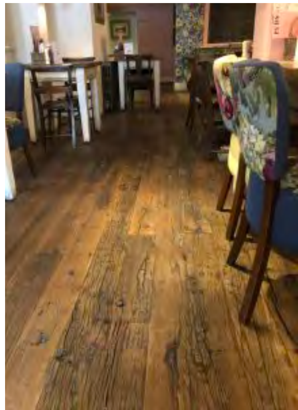
The floors all have a resin damp proof membrane beneath them, to prevent the water rising from underneath.
