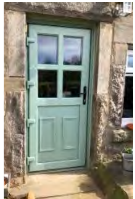
Flood door fitted.
