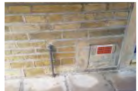
Walls were repointed and coated with a water proof spray and self-closing airbricks fitted.
