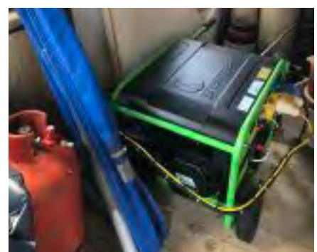
They have another pump and generator as a backup.
