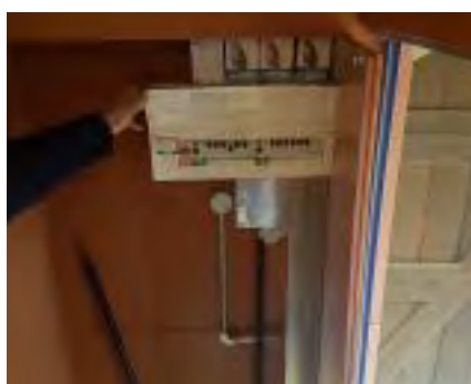
Raised electrics with with drops from ceiling level.
