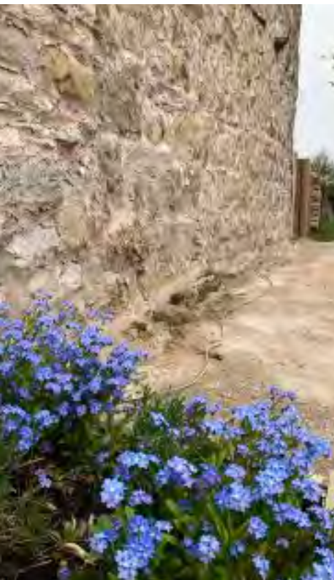
The gable end of the property has been under pinned and repointed.
