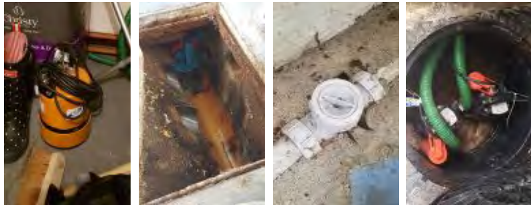
Puddle sucker, non return valves added to all the pipe work and sump pumps in the outhouse.
