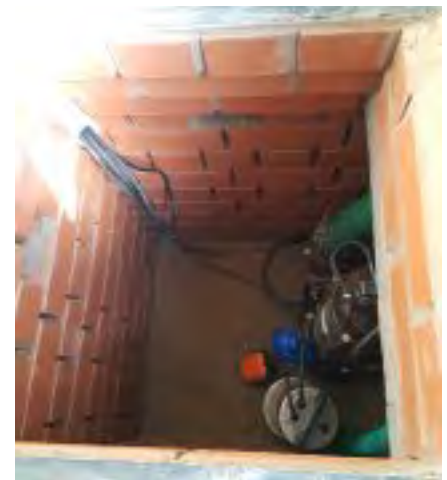
Two sump-pumps in lounge.
