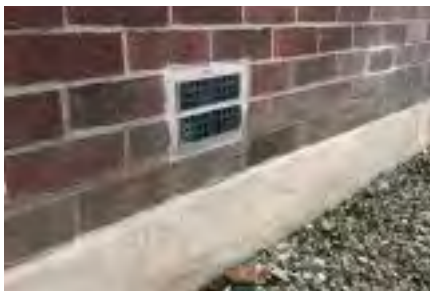
Self-closing air bricks and waterproof rendering was applied underground to the foundations and 30cm above ground.
