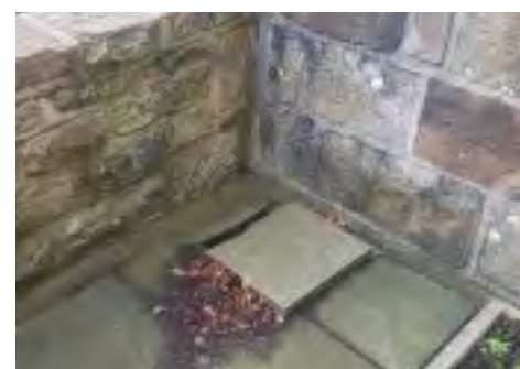
Sump created, into which powerful submersible pump can be dropped when flooding commences.
