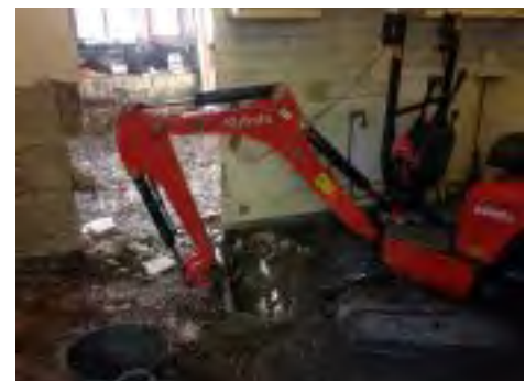
The rebuild involved excavating and 'tanking' the whole of the ground floor
